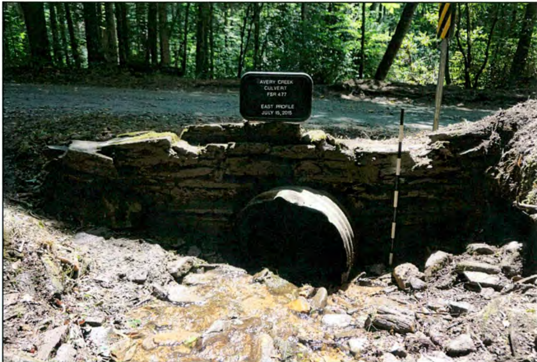
Figure 16. Profile view (with scale) of headwall at Avery Creek Road culvert. View to east.
