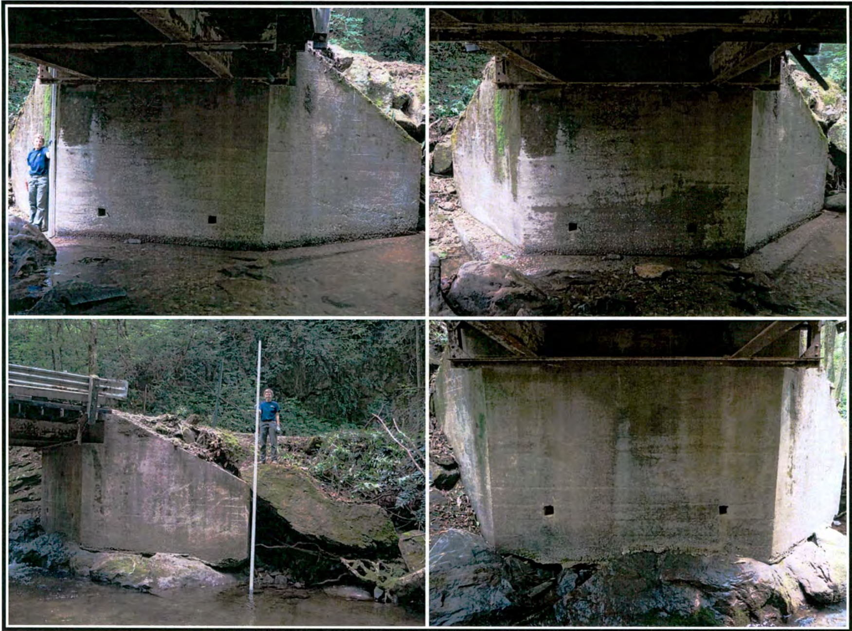
Figure 10. Overview and close-up photographs of the concrete abutments at Bridge 140-1.5: a-b) north abutment, view to northwest; c) south abutment, view to east; south abutment, view to southeast.
