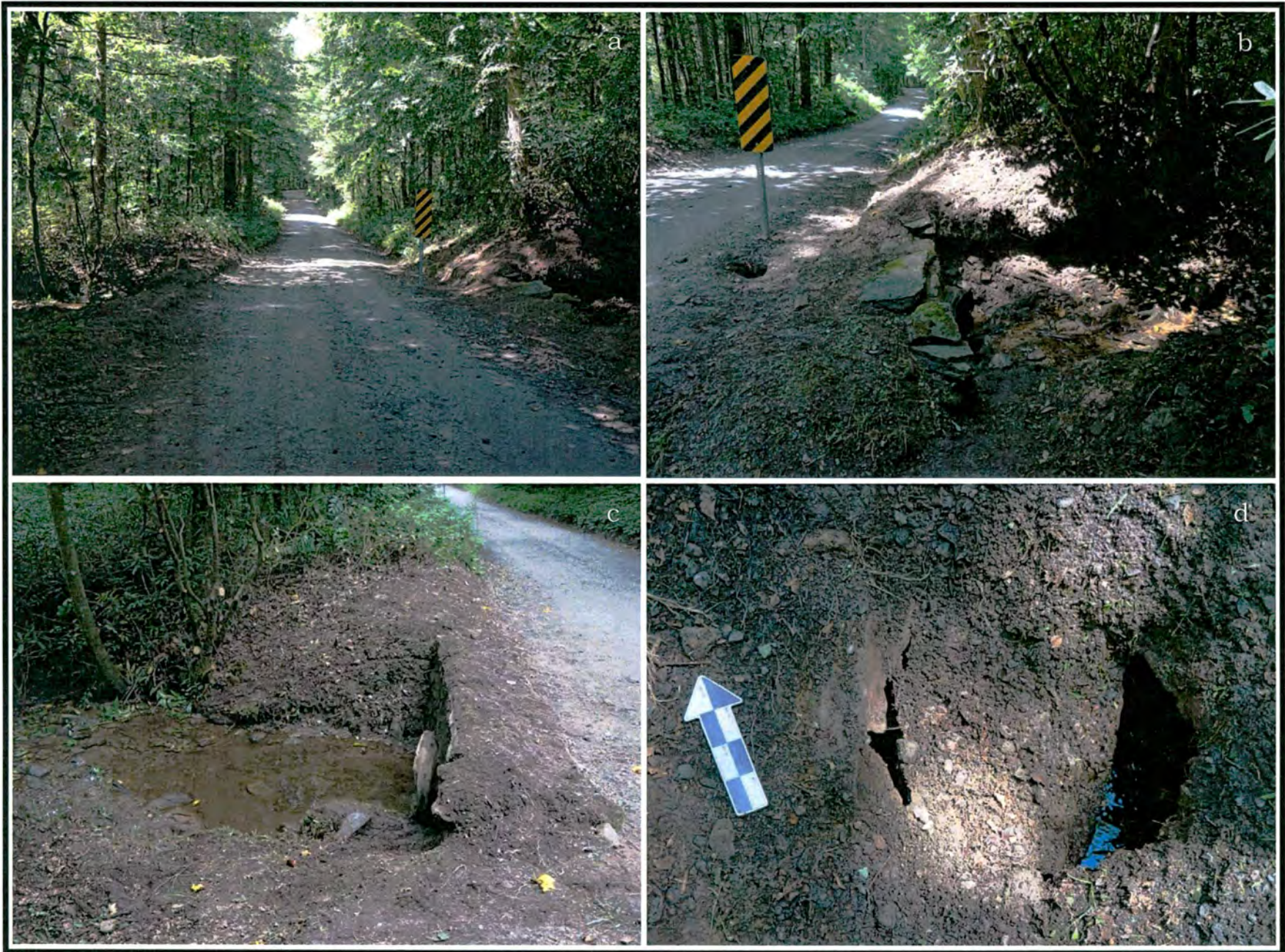
Figure 14. Overview photographs of the Avery Creek Road culvert on FSR 477: a) view to south/southwest; b) headwall & breach in culvert, view to south; c) outflow wall, view to southwest; close-up of breach in steel culvert/FSR 477, view to northeast.
