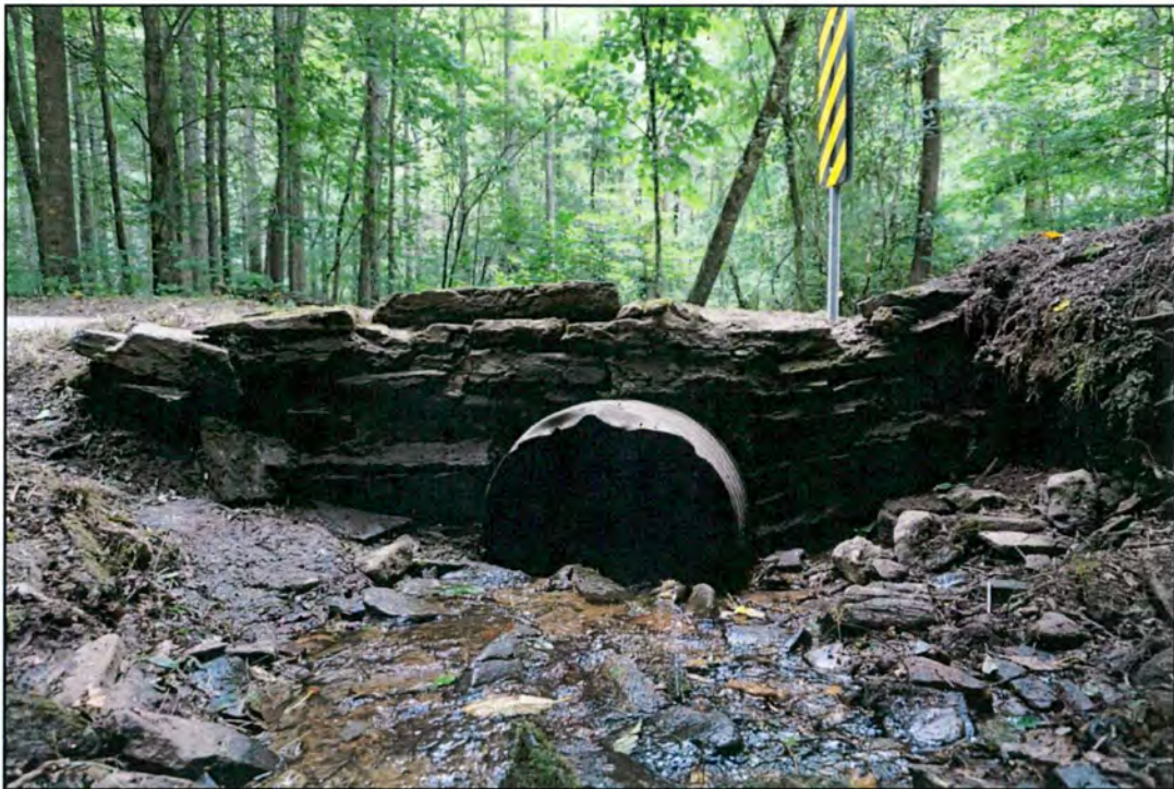
Figure 17. Profile view of headwall at Avery Creek Road culvert. View to east.
