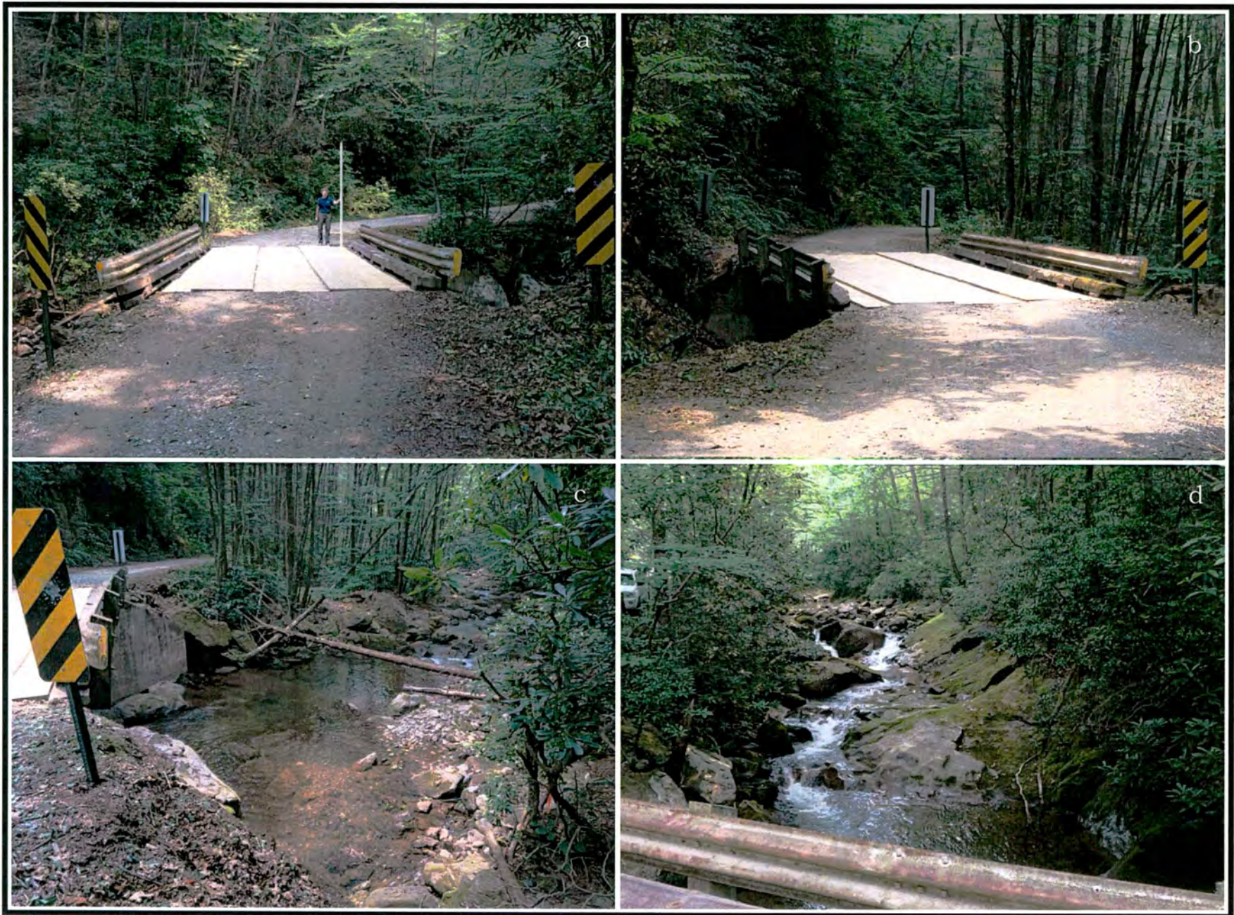
Figure 5. Overview photographs of Bridge 140-1.5 and Courthouse Creek: a) Bridge 140-1.5, view to northwest; b) Bridge 140-1.5, view to southeast; c) upstream portion of Courthouse Creek, view to southwest; d) upstream portion of Courthouse Creek; view to northeast.
