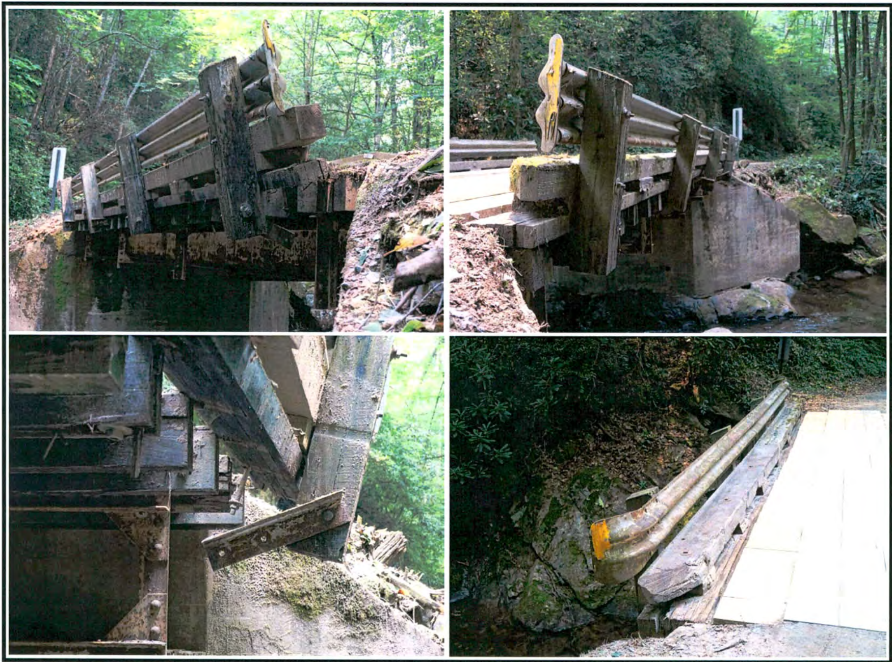
Figure 13. Overview and close-up photographs of the wood and steel railings at Bridge 140-1.5: a) south railing, view to north; b) south railing, view to southeast; c) close-up of broken support bracket on south railing, view to southeast; and d) north railing, view to southeast.
