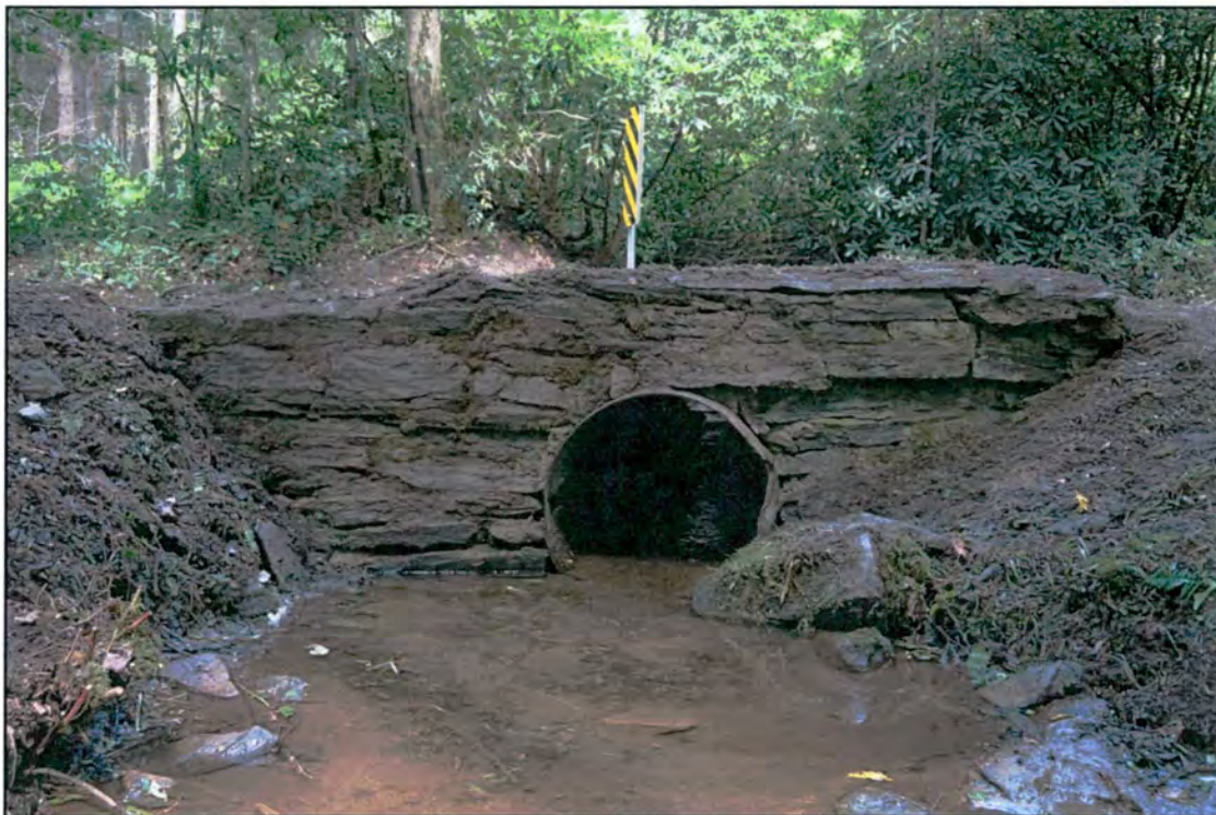
Figure 20. Profile of outflow wall at Avery Creek Road culvert. View to west.
