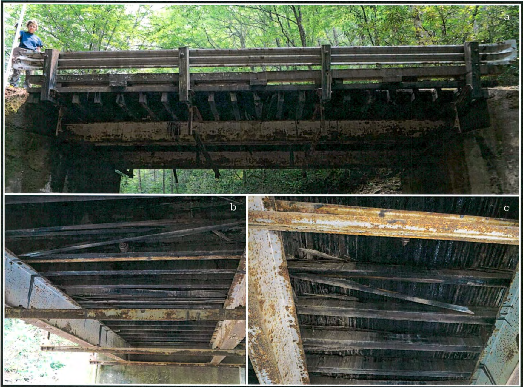
Figure 12. Overview photographs of the steel girders, steel angle brackets, wooden transverse joists, and laminated decking at Bridge 140-1.5: a) view to northeast; b) view to northwest; and c) view to southeast.
