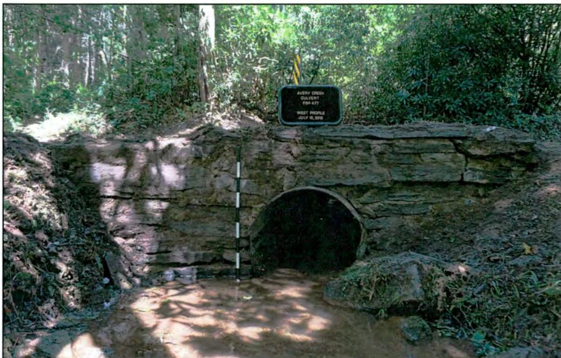
Figure 19. Profile view (with scale) of outflow wall at Avery Creek Road culvert. View to west.
