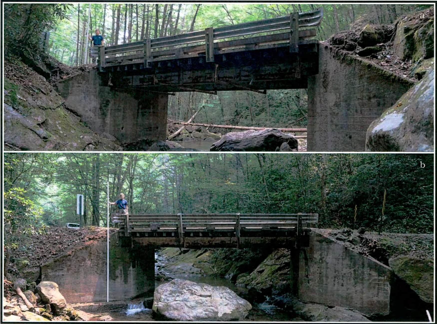
Figure 6. Overview photographs of Bridge 140-1.5 on Courthouse Creek: a) view to southwest; b) view to northeast.
